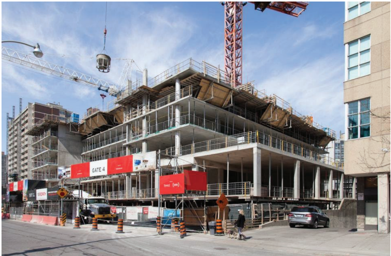
The 155 Redpath site in mid-May, looking northeast from Redpath Avenue, image by Jack Landau
